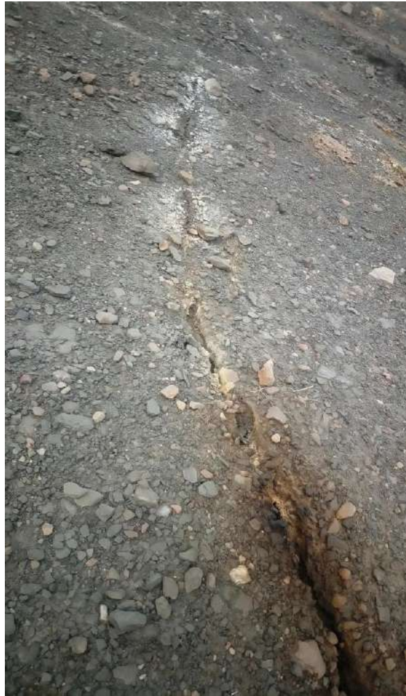
Figure 20: Fume cracks in the Bhulanbarari area.
