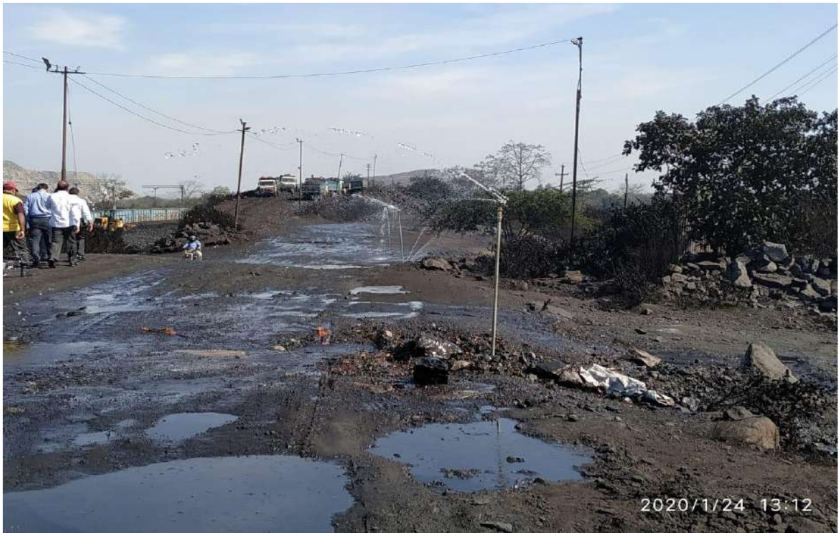
Fixed type water sprinkler system at Railway siding
