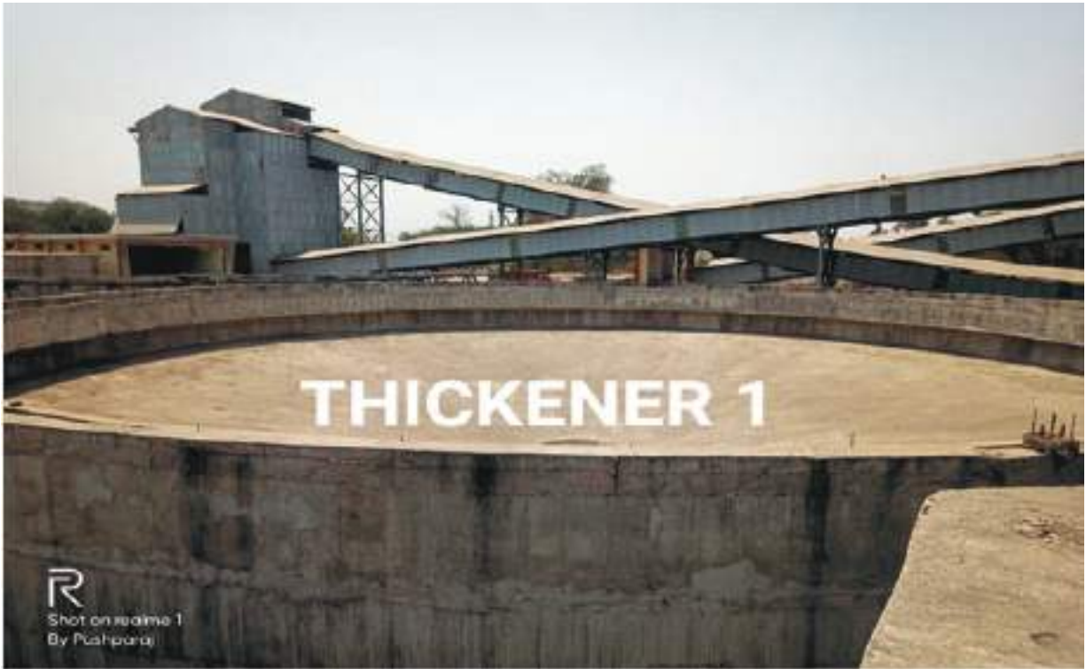
Thickener-1 2.0 Mtpa BHOJUDIH WASHERY
