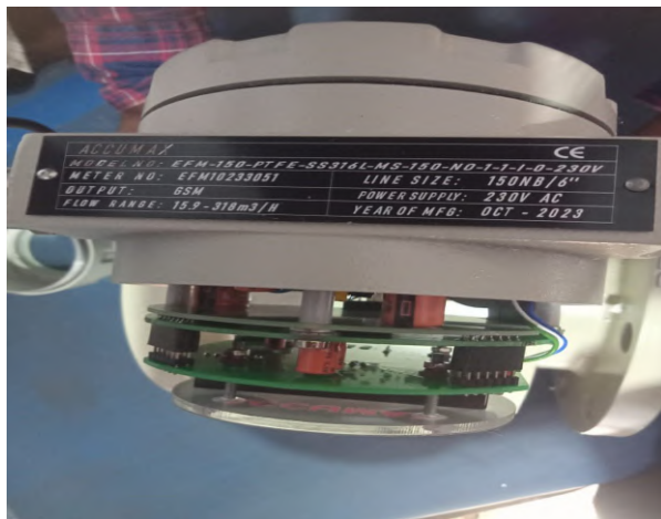
ETP in Central Hospital, BCCL
