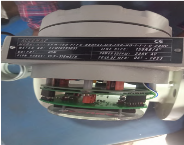
ETP in Central Hospital, BCCL
